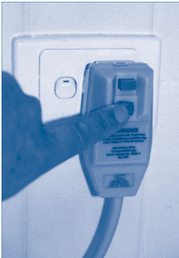
Demonstration of RCD push-button test
